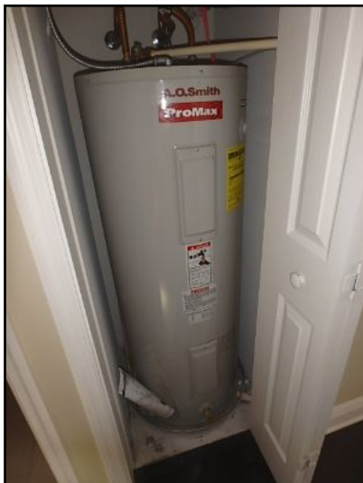
Noted that the water heater has an odor (bacteria), recommend flushing out the tank
