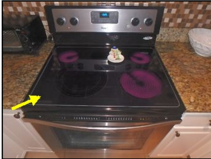
left front burner has crack and does not operate
