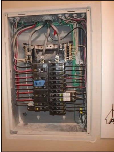
No major system safety or function concerns noted at time of inspection at main panel box.
