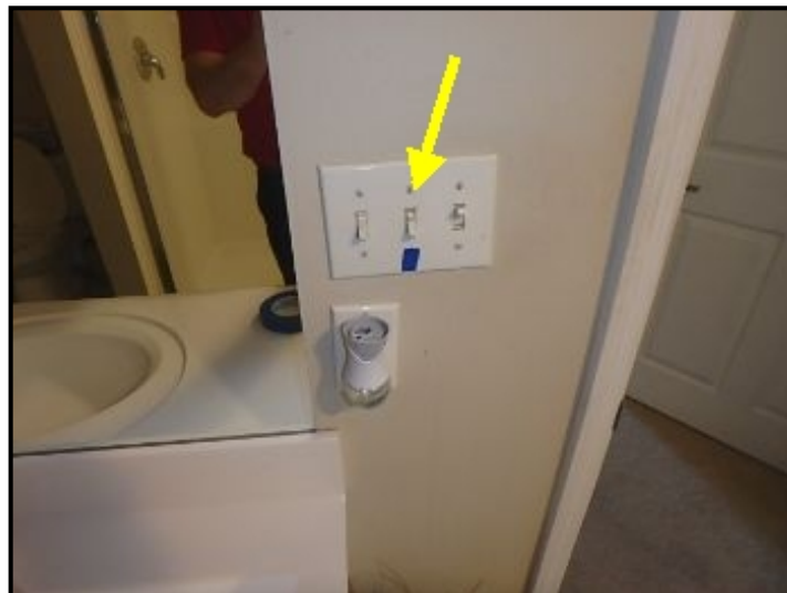
Middle switch in Master bathroom is faulty, loose contacts.
