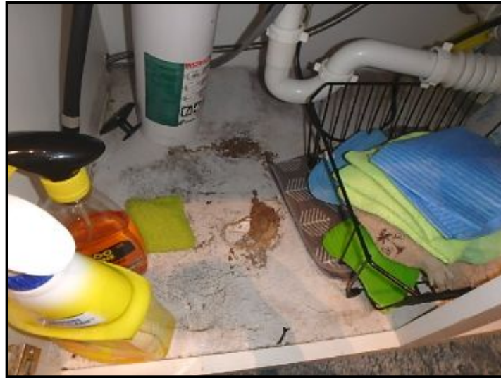
past moisture damage noted under kitchen sink.
