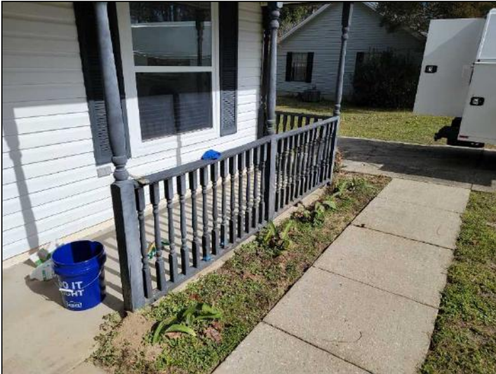
Rotted Wood numerous spots on front rails.
