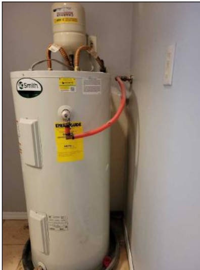
TPR Valve discharge tube is routed upwards. Needs to flow down
