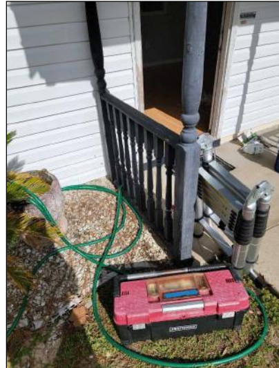
Rotted Wood numerous spots on front rails.
