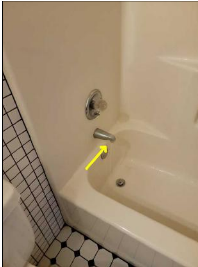
Shower diverter does not fully engage. Recommend repair. Guest Bathroom
