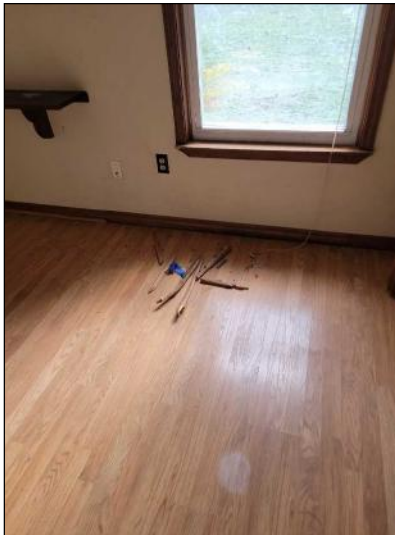
Toe molding damaged in numerous spots
