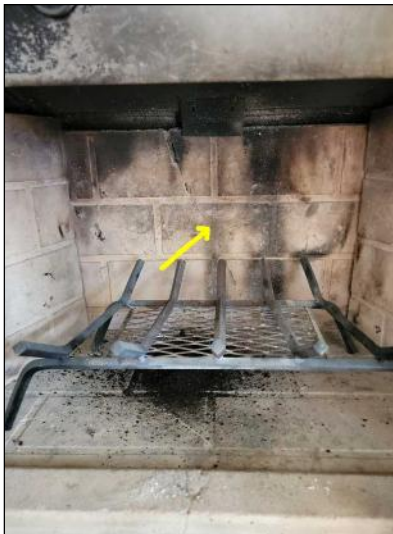
Fire brick cracked on rear. Recommend repair
