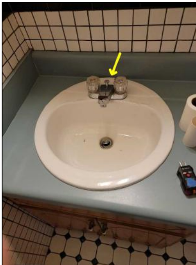
Stopper is missing/inoperable. Recommend repair. Guest Bathroom
